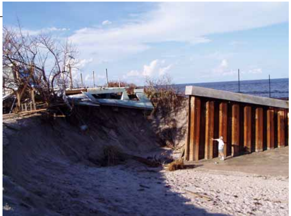
Over 50 feet of accelerated dune recession around the southern "return wall" of the Wabasso seawall, just south of the Archie Carr National Wildlife Refuge. Note the complete loss of two of the homes this wall was built to protect.
